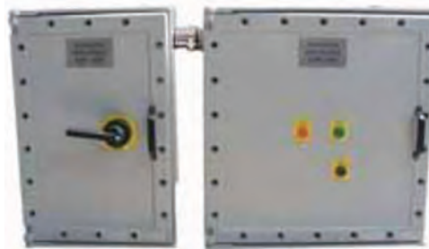
160kW Motor Starter Protected by Manual Circuit Breaker Kompak Şalter Korunmalı 160kW Motor Starter
